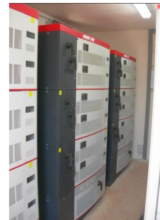
No. 3 Inverter Power one Aurora PVI-330.0-TL-IT
