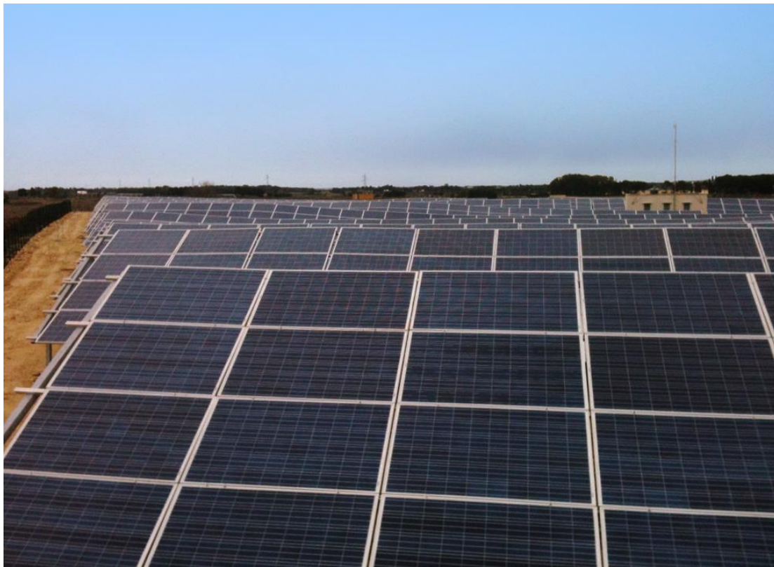
Complete view of installation
