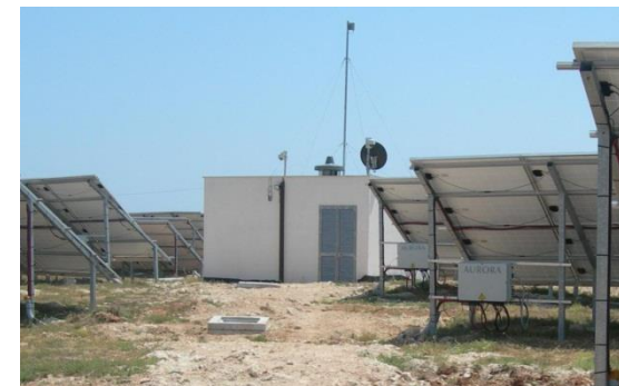
Detail of installation and inverter station
